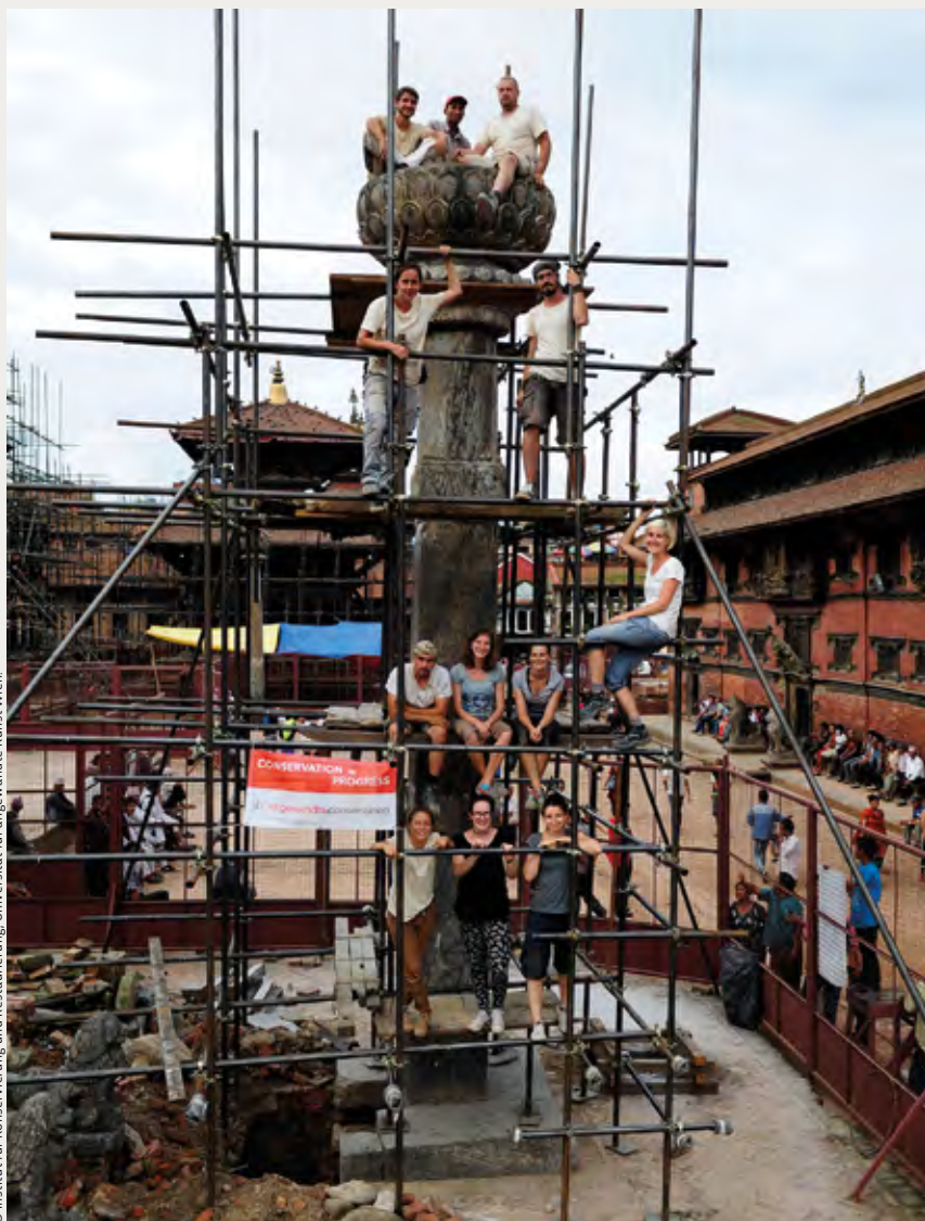
It proved possible to re-erect the collapsed Pillar of King Yoganarendra Malla on Patan Durbar Square just one year after the horrific earthquake in Nepal
